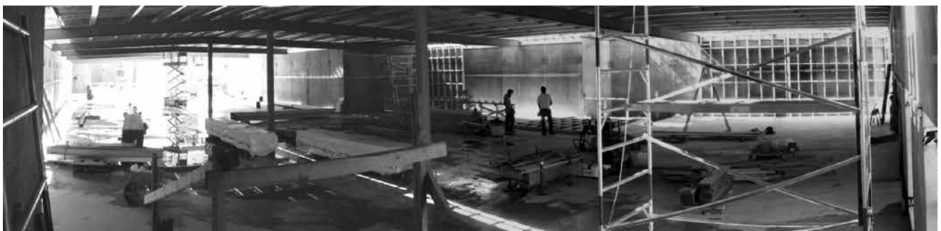
A panorama of the interior of the new collection store earlier in the construction.
